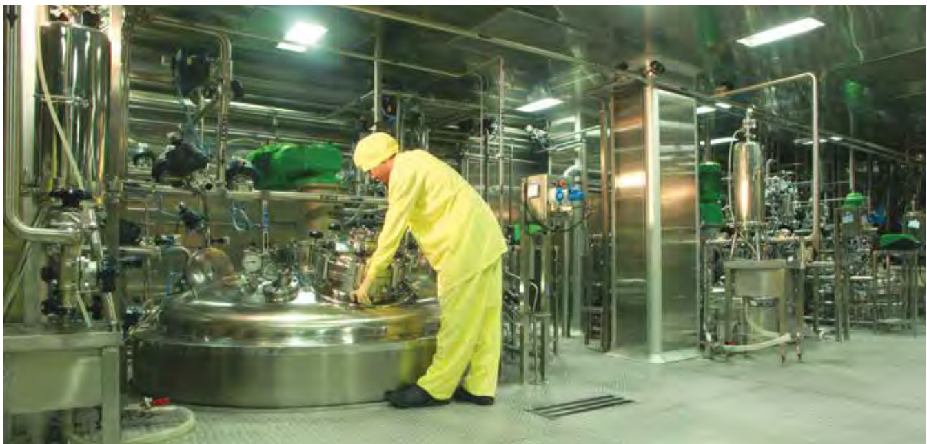
Inside of a Vaccine production plant
