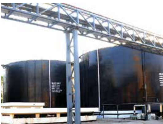
Fig. 3.8 Molasses storage tank
